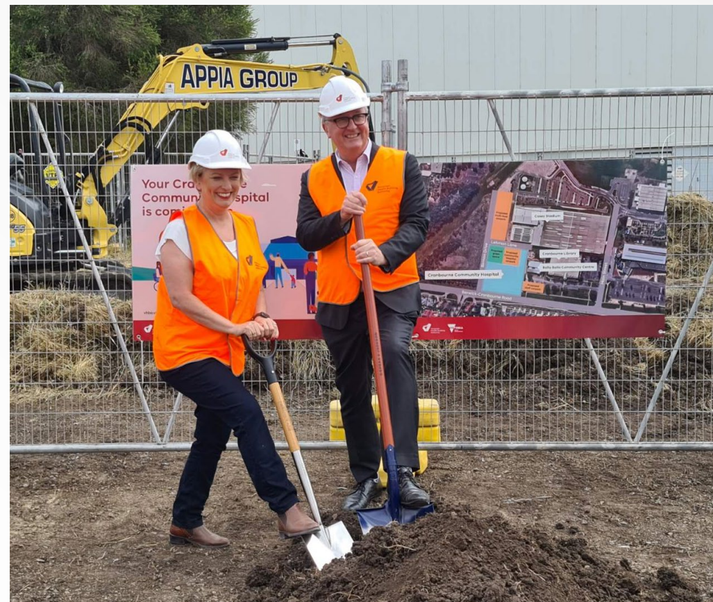
Pauline Richards and Martin Foley Turning the Soil for the New Cranbourne Community Hospital 21 Dec 2021
